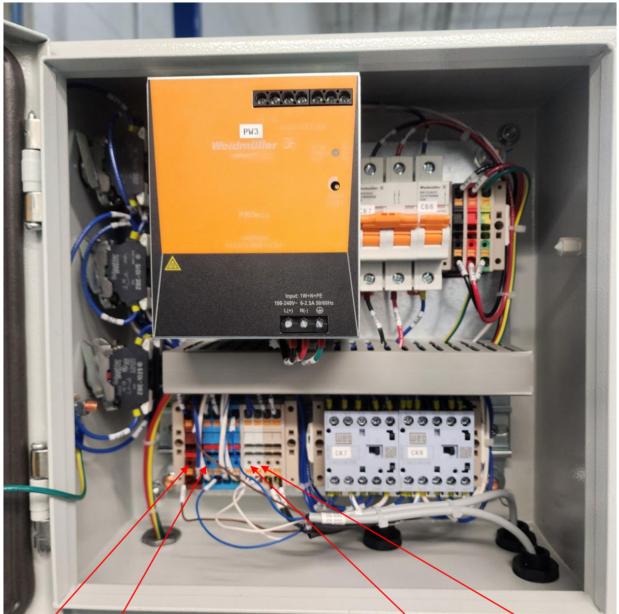
Figure 9 DC Power Supply Voltage Check
